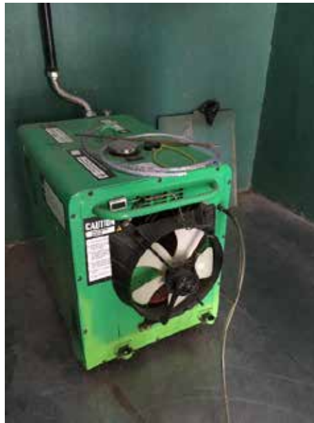
Figure 4. Generator (Photographed by the authors)
