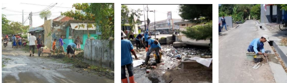
Figure 4. Routine Maintenance by the Community (left), by Local Government (middle) and by Drainage Repair Worker.
